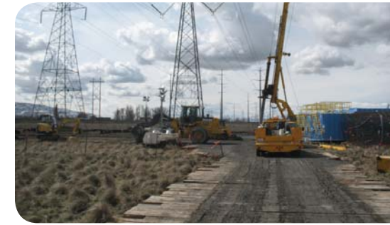
Local Project Success: Legacy Utility Line Construction Removable roadway placed on ground to facilitate access for large equipment so damage to site is minimized. Photograph by Eric McCulley
