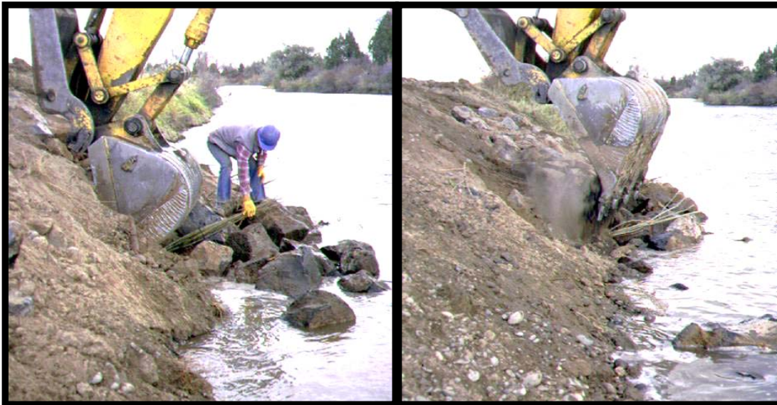
Figures 6 and 7: Excavator bucket is pushed into the streambank above the rock riprap in the keyway trench. Operator lifts the soil up (without pulling the bucket out) to create a small hole underneath. Another person shoves the willow bundle into the hole and the operator pulls the bucket straight out and the soil drops on to the bundle.
